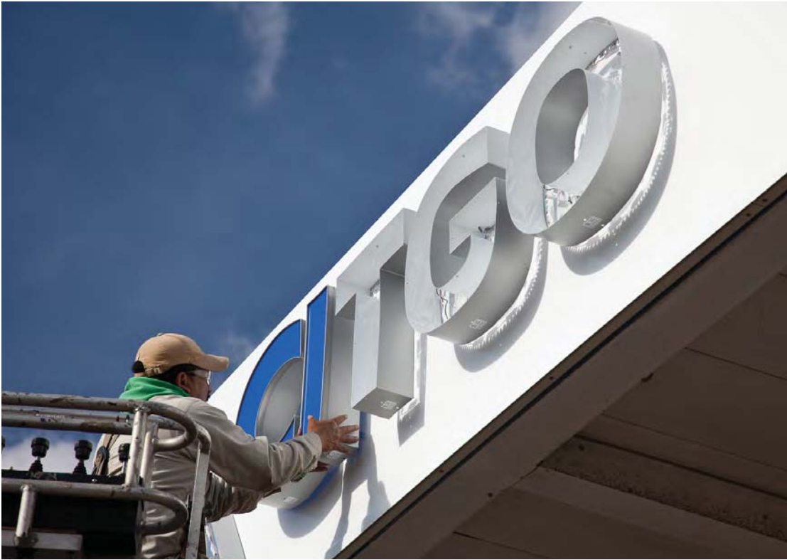
Installing the primary CITGO channel letters. Note the spacers that provide the rear halo effect on these channel letters.
