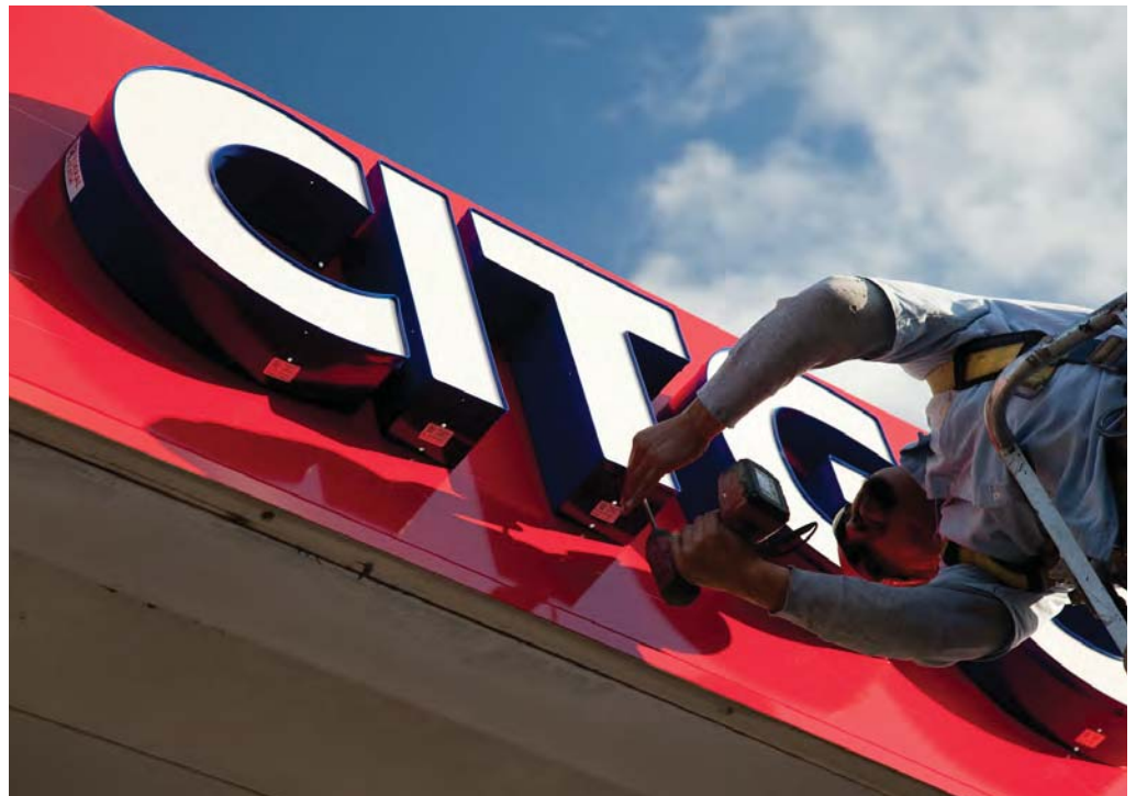
Installing the faces of the white secondary CITGO channel letters. Note that they are flush mounted and the sides of the channel letters are blue.
